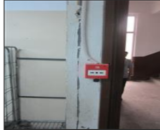
Photo of the inside of the main production hall fire alarm button.JPG
