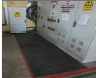
Photo of the inside of the main production hall electricity panel (2).JPG
