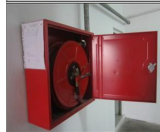
Photo of the inside of the main production hall fire hose.JPG
