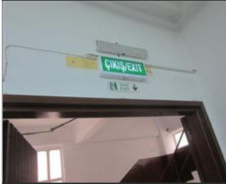
Photo of the inside of the main production hall exit sign & emergency light.JPG
