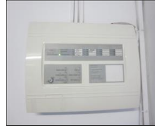
Photo of the inside of the main production hall fire alarm control panel.JPG
